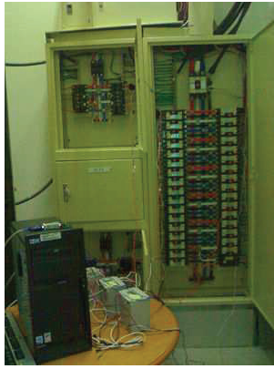
Figure 6: PA-310, electric panel and server
